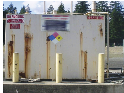
Rusted Steel fuel tank
